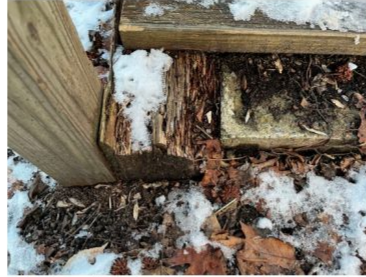
Existing conditions / rotten areas
