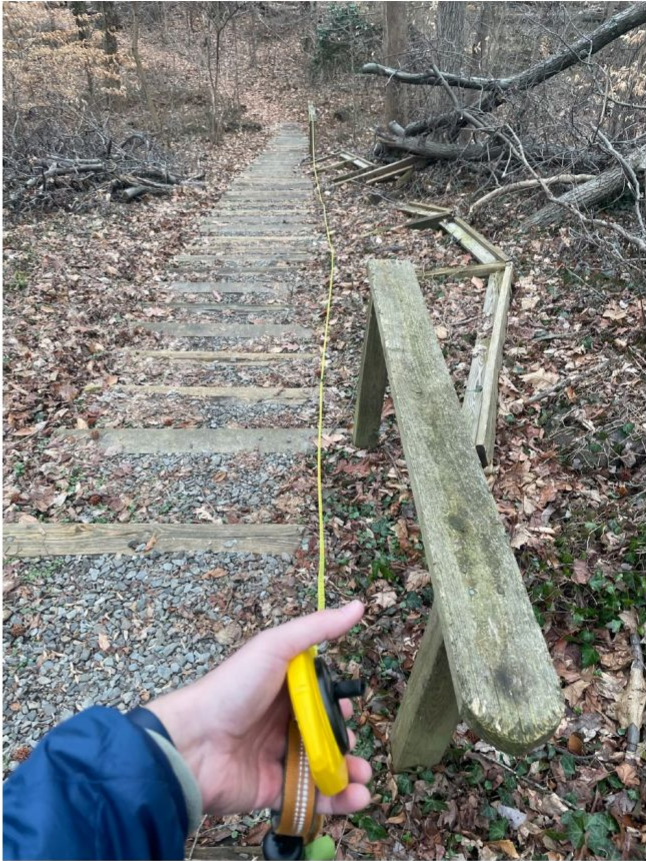
Existing conditions / damaged handrail
